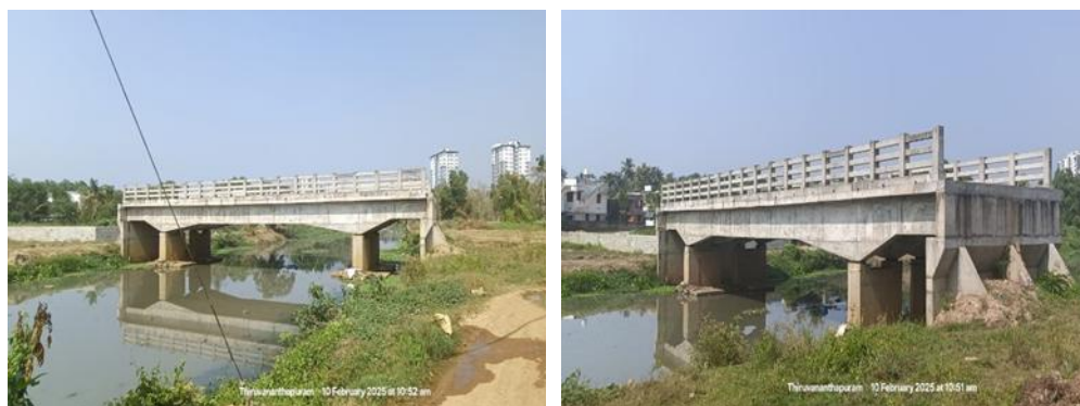
Figure 9: Bridge constructed across Amayizhanjan Thodu found isolated due to non-acquisition of adjoining private land for the approach road.
