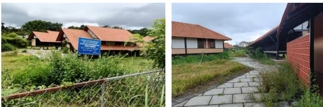
Figure 7: Valliyoorkavu Market and Exhibition Space building found abandoned and structurally deteriorated.
