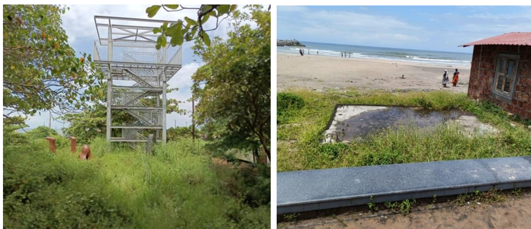
Figure 1: Tower at one end of the zip line and partially completed piling work for the second tower at the other end lying abandoned.
