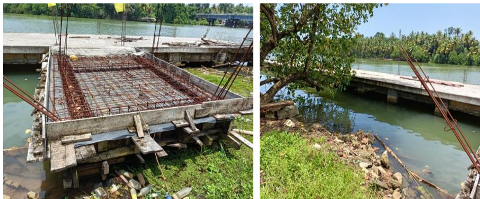
Figure 10: Abandoned House Boat Terminal at Monroe Island. JPV revealed rusted steel bars and incomplete landing facilities.
