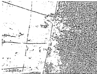
Fig 6. Construction joint in dome slab through which seepage of water is observed
